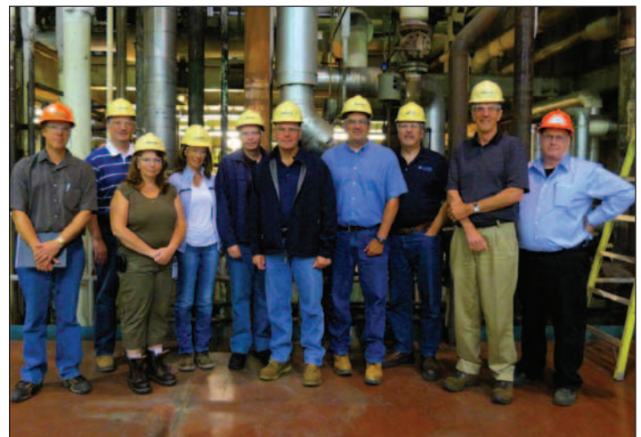
Union Gas representatives toured Thunder Bay GS as plans progress to repower the station from coal to natural gas.
